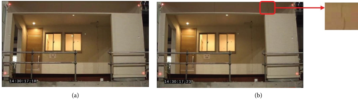
FIGURE 15: The example frames with (a) closing ( t = 2.6 s) and (b) opening of the tiny crack ( t = 2.8 s).
