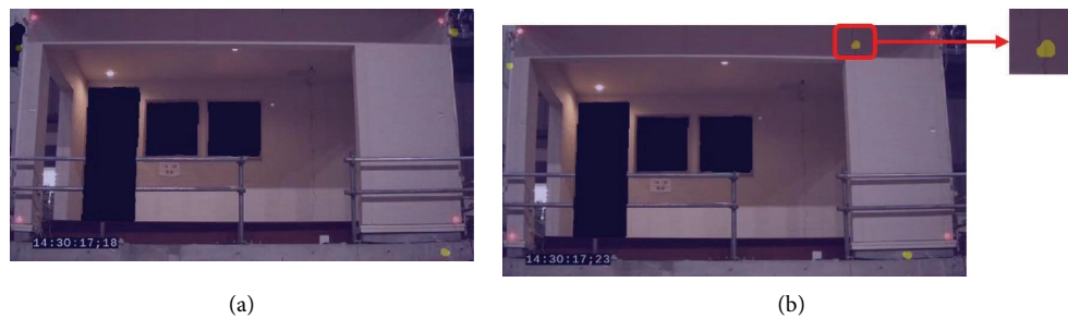
FIGURE 19: Results of feature enhancement for the tiny crack: (a) closing of the crack ( t = 2.6 s) and (b) opening of the crack ( t = 2.8 s).
